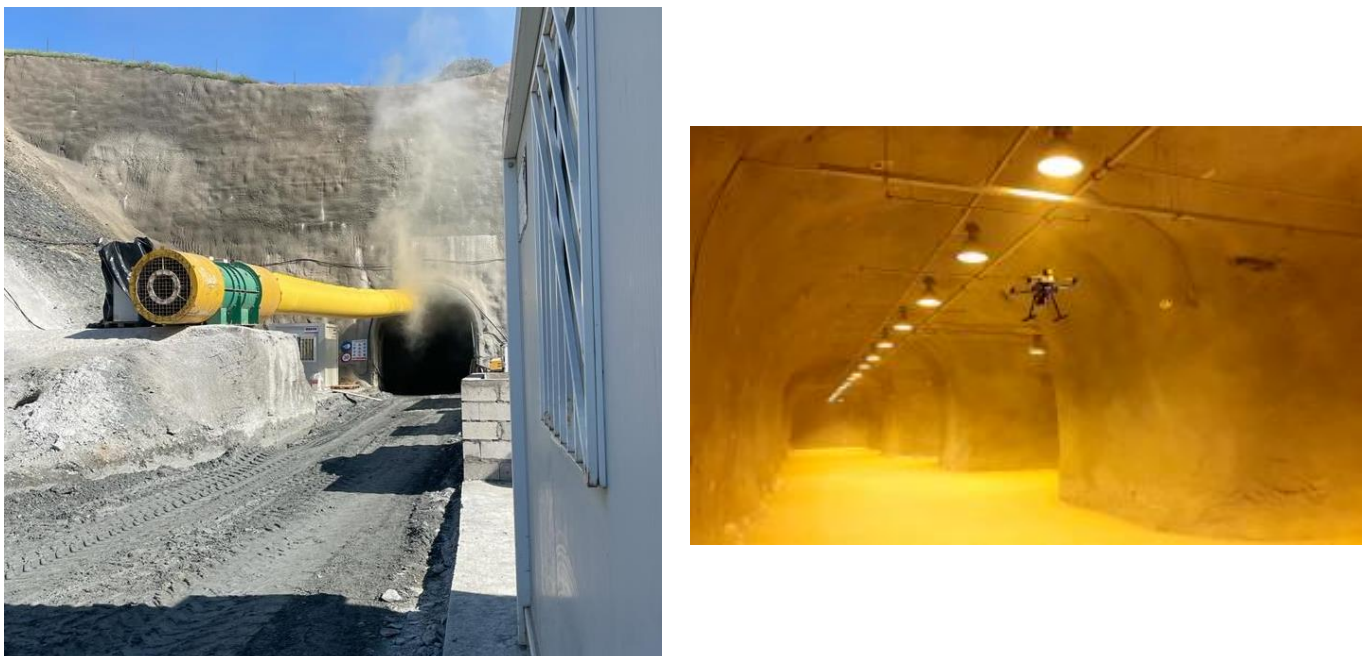
Figure 11. Tunnel access (Seville, Spain) and Lavrion Technological and Cultural Park (Attica, Greece).
