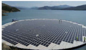
Figure 21. Banja FPV Project in Albania.
