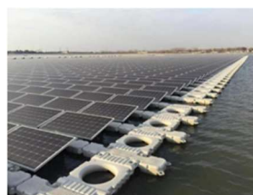
Figure 11. The 150-MW floating PV in Huainan, Anhui Province, China [20].
